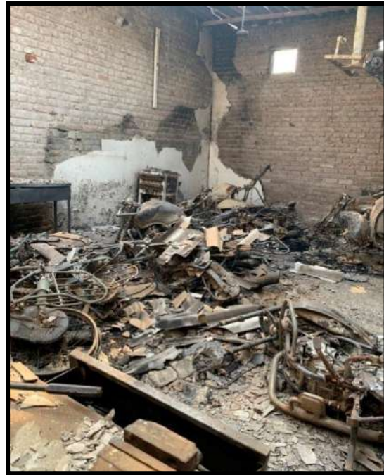
Burnt shop of Bhandari Services
