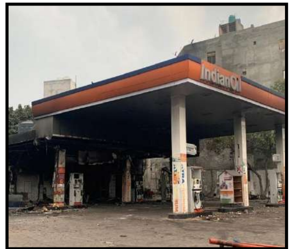
Burnt Petrol pump of Bhajanpura
